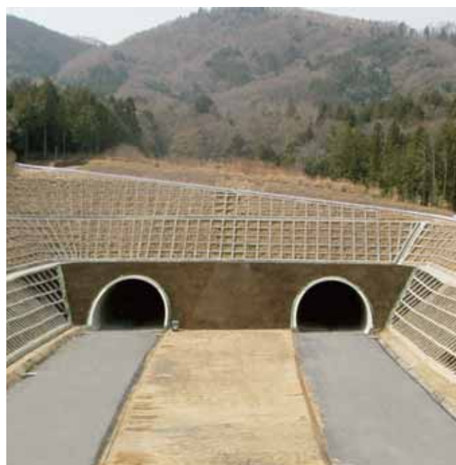
Construction on Iwase Tunnel East, Kita-Kanto Expressway Location: Ibaraki, Japan Client: East Nippon Expressway Co., Ltd.
