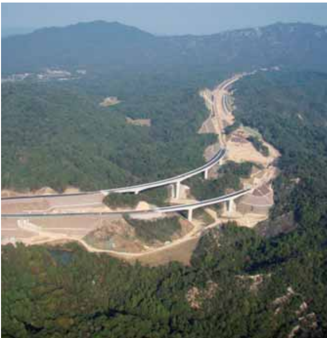
Construction on Otsu Junction, Second Meishin Expressway Location: Shiga, Japan Client: Kansai Branch Office, West Nippon Expressway Co., Ltd.
