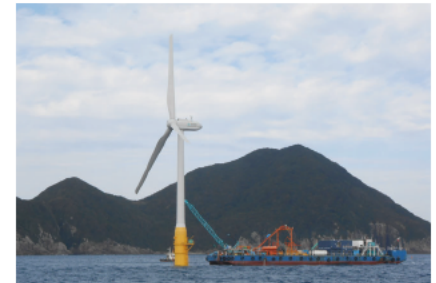
6. To complete the installation, mooring chains and submarine cables are connected to the turbine at the installation site.
