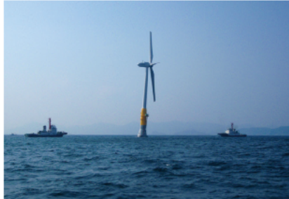
5. After its completion, the wind turbine is towed from the assembly site in the sea north of Kabashima to the installation site.
