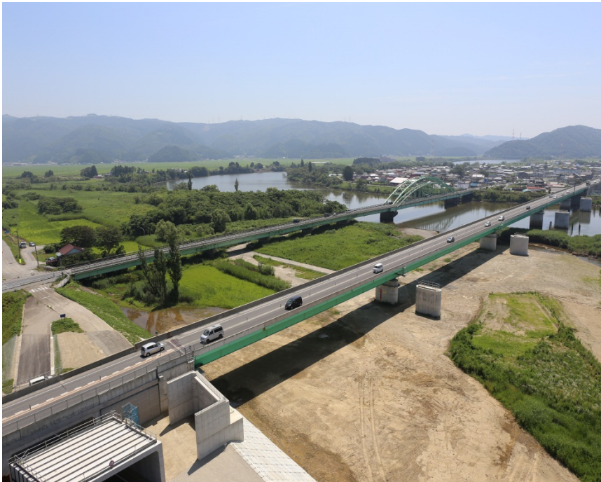
Yamato Ishinomaki Road substructure work, Tohoku Regional Development Bureau, Ministry of Land, Infrastructure, Transport and Tourism
